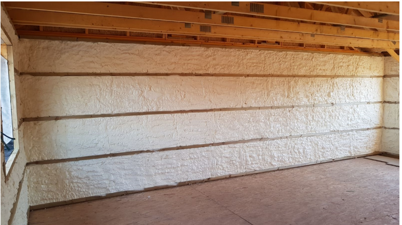
Figure 2 - the Product built up between counter battens over timber studs to minimise thermal bridging and seal the joints in the timber frame
