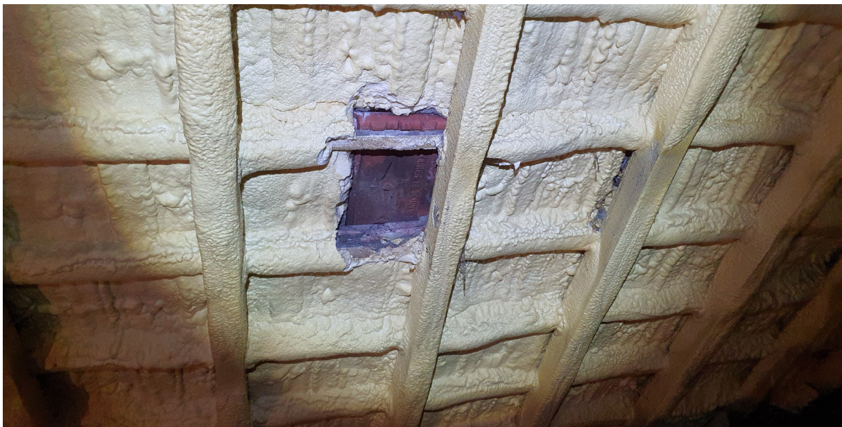
Figure 1: Spray foam used to stabilise a failing roof cover; a thin coating with limited heat retention but significant water problems
