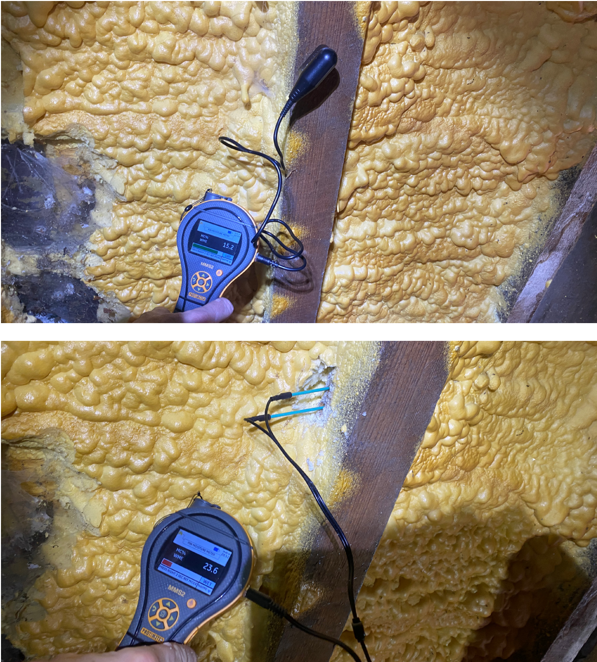
Figure 3: Spray foam insulation can make it difficult to identify problems to the roof because the timbers can be 'dry' on their exposed, visible surface but 'wet' behind the spray foam
